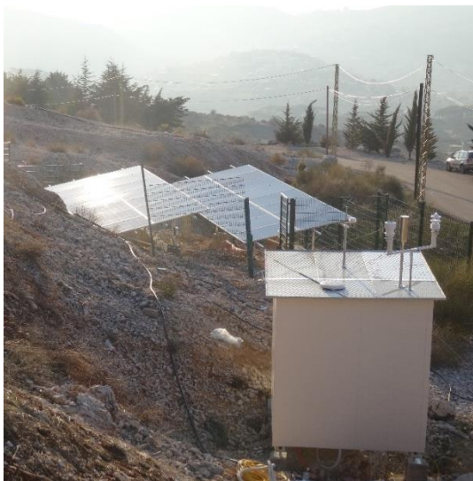
Figure 10: A newly installed air quality monitoring station in Barouk, Mount Lebanon Source: StREG resources
